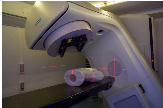
Figure 1. Radiation-therapy room with gantry and positioning lasers (red)
